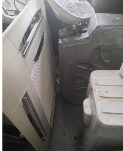
1 – Ceiling Cassette Aircon with condenser
